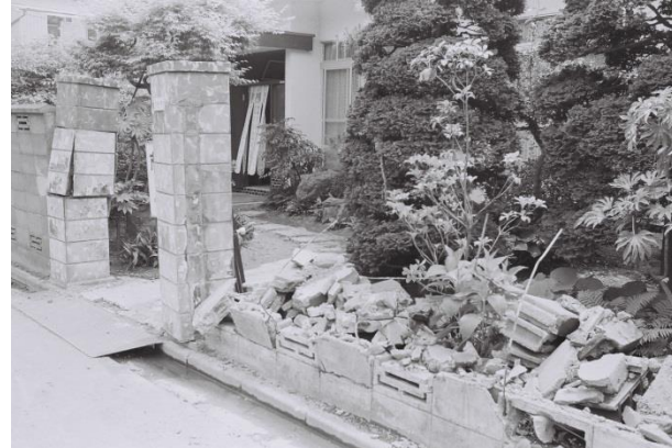
Destroyed brick walls
