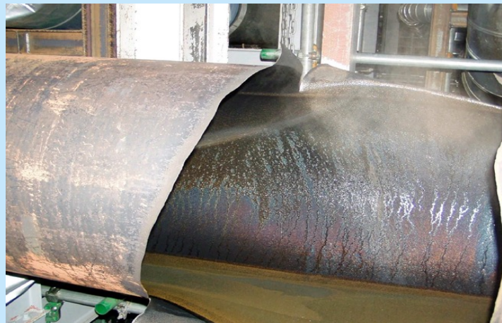
Pipe breakage accident in Mihama power plant in Japan (2004.8.9)
